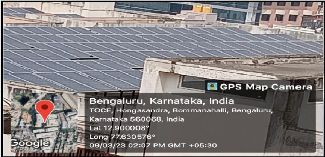
Overview of Solar Panel
